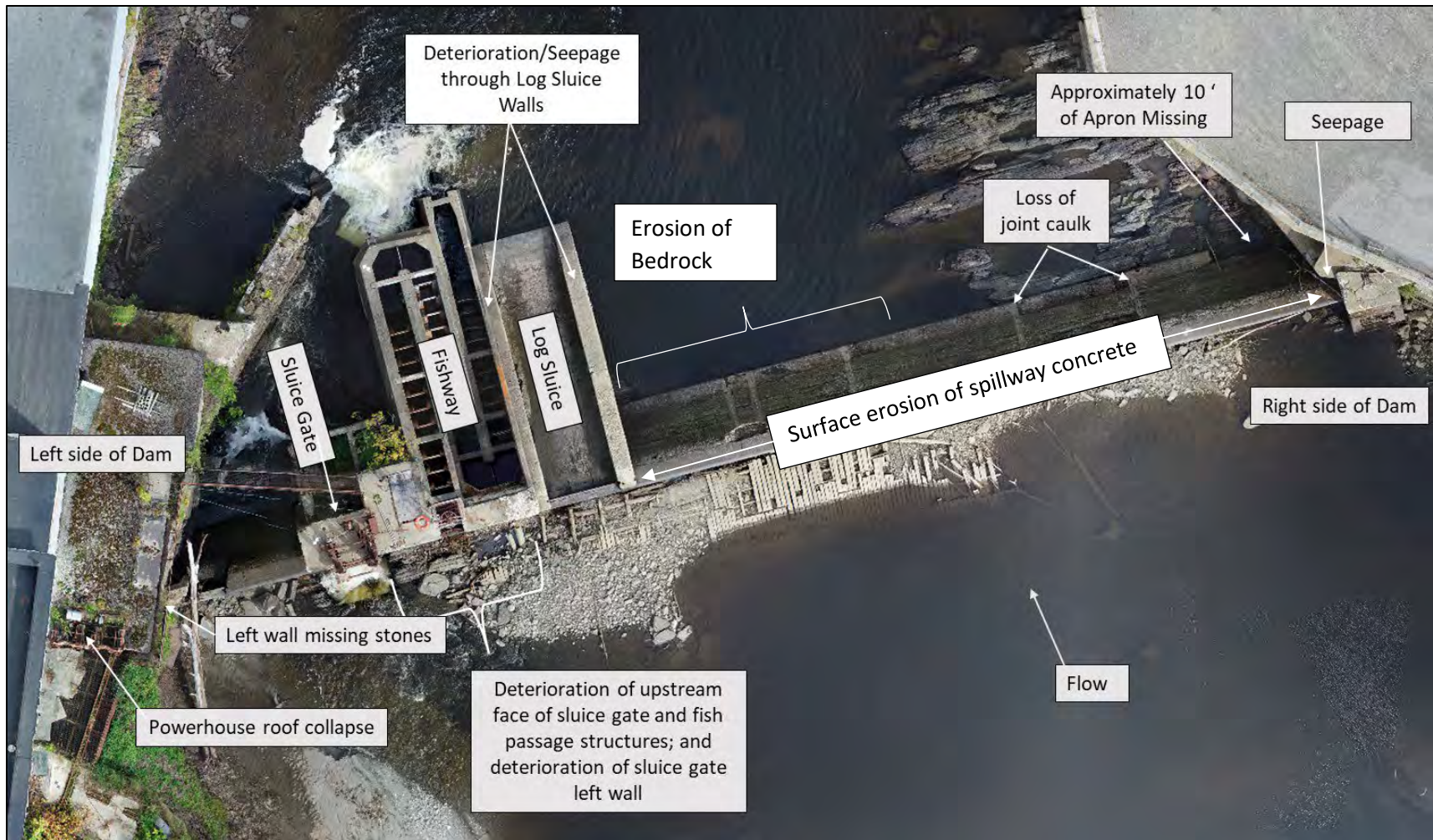
Figure 2.1-1. Aerial Image of Dam with Structural Deficiencies Labeled
