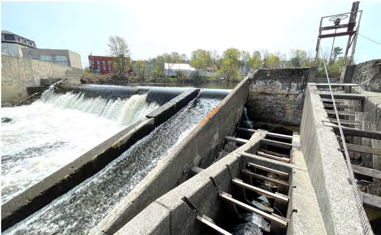
Figure 28. May 2023 photo showing condition of spillways and fishway prior to being opened for the year, including leakage at the base of the log sluice into the fishway.
