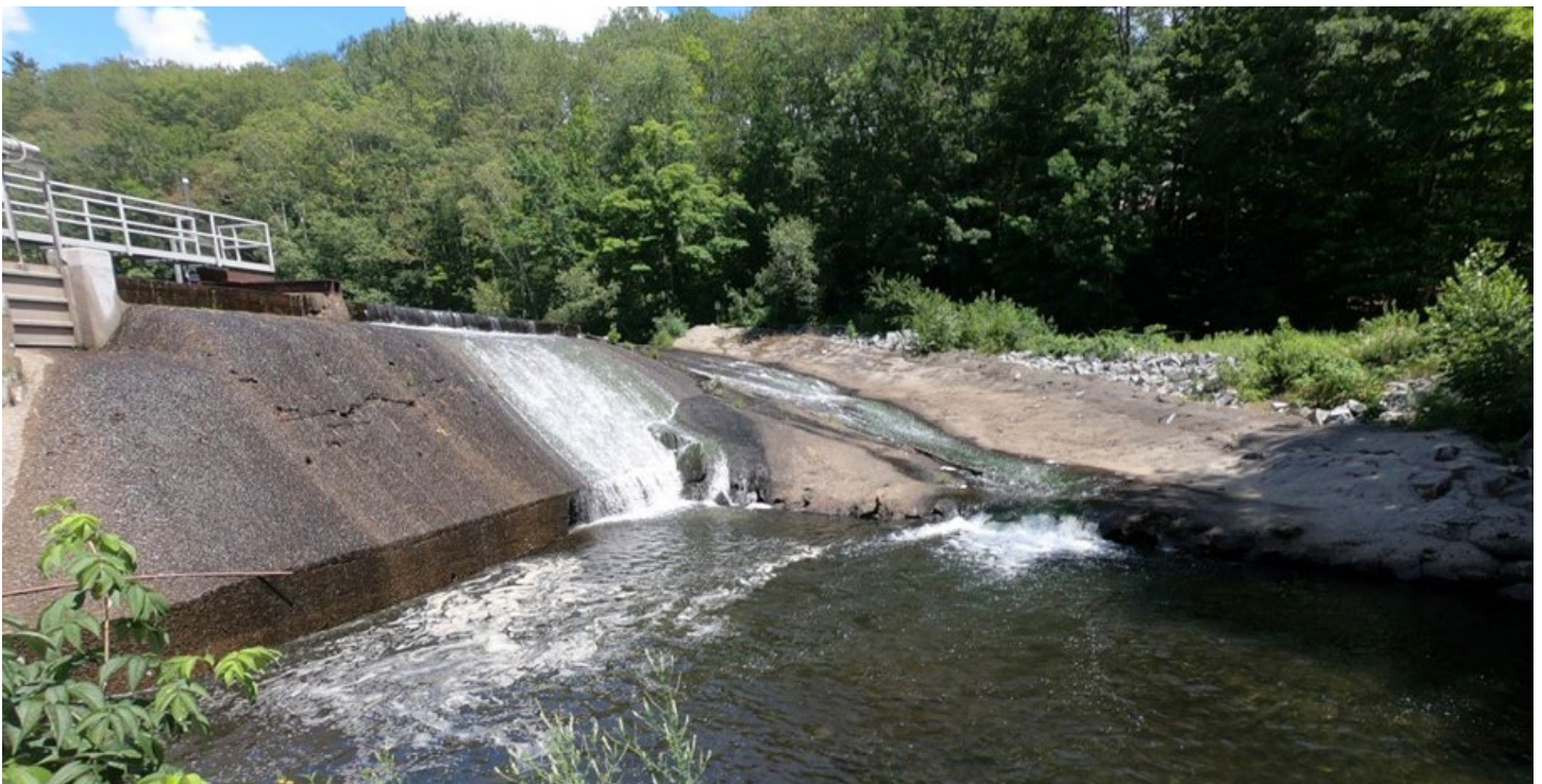
Technical and naturlike fishway alternatives to restore fish passage while maintaining upstream lake levels were developed for Scabright dam, a recently retired FERC-exempted hydroelectric facility.
