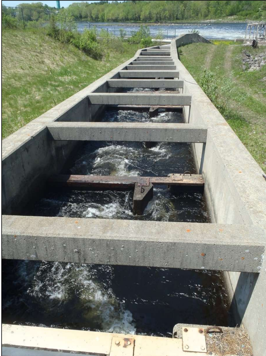
Figure 14. Vertical slot fishway at West Enfield (photo credit: USFWS). This type of technical fishway is considered under Alternatives M1 and L1.
